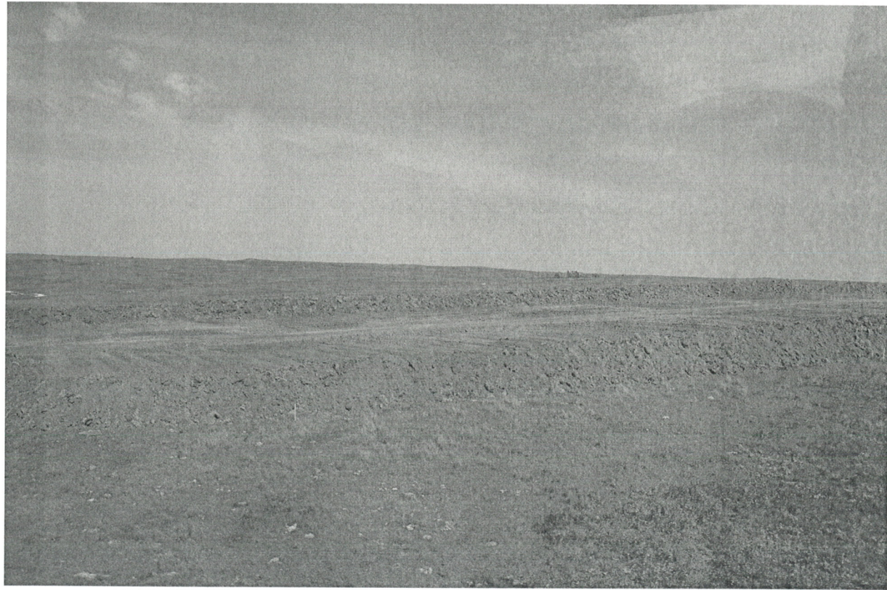
Figure 4. Photograph of the Dakota Access Pipeline construction corridor inventory area showing stripped surface and stockpiled topsoil berms along the lateral margins.
